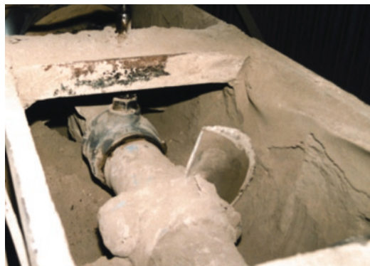
Hanger bearing on a gypsum scroll conveyor
