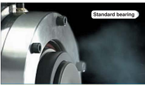
A large amount of oil mist passes through the bearing, contaminating the working environment.
