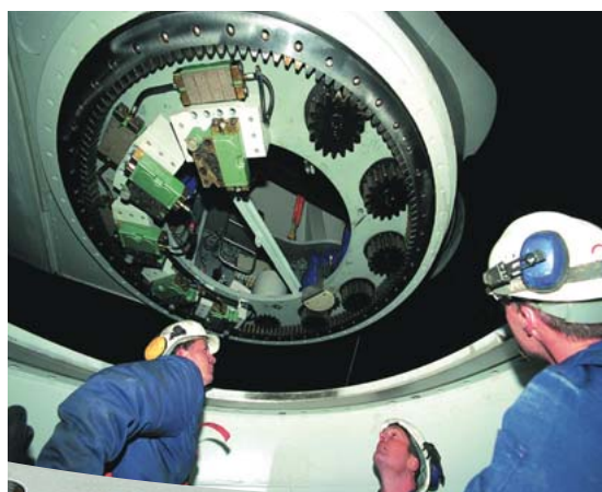
The nacelle with Yaw Bearing already attached, is lowered onto the turbine tower.
