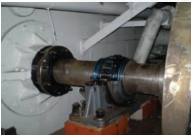
Cooper bearing on a marine generator drive during inspection
