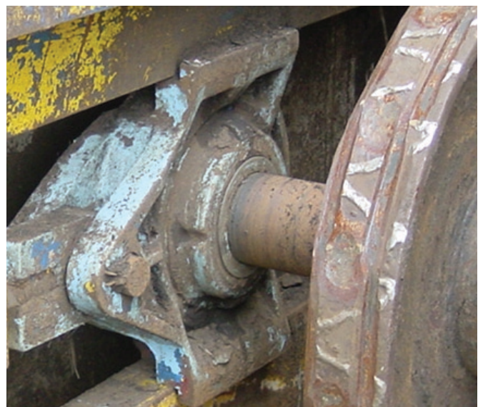
Cooper tension take-up unit in a trapped location on a sugar mill conveyor
