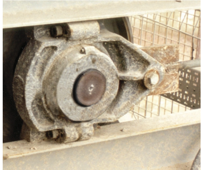
Typical Cooper tension type take-up unit in an aggressive quarry environment
